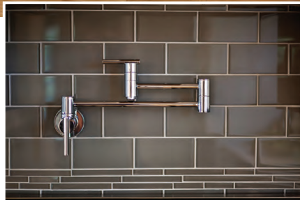
At right: A modern luxury in the kitchen is the pot filler installed above the gas range, making filling stock or pasta pots a breeze.
